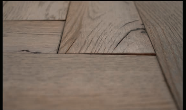
SURFACE CHECKS / OVER-WOOD
