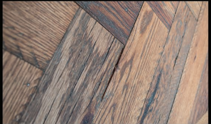
NAIL HOLES, SURFACE CHECKS, OVER-WOOD
