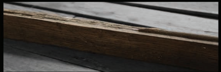
NAIL HOLES, SURFACE CRACKS, BROKEN TONGUES
