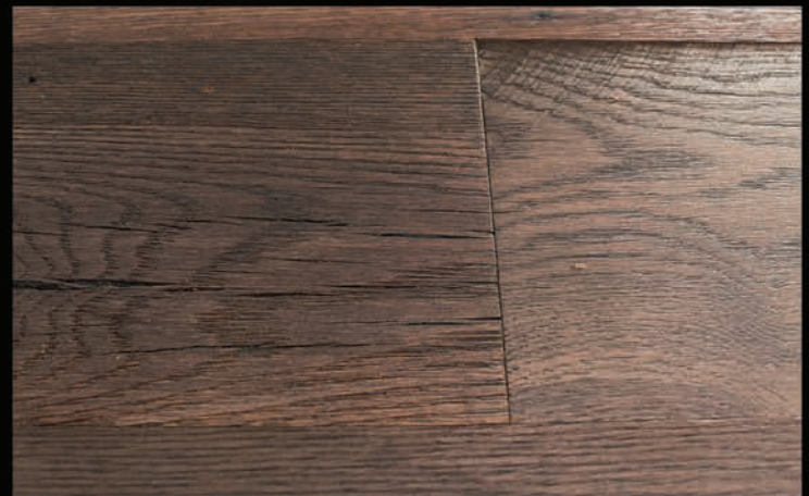
NAIL HOLES, SURFACE CHECKS, OVER-WOOD
